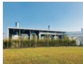
View of the Suzhou air purification system
