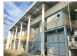
Partial view of the Suzhou air purification system
